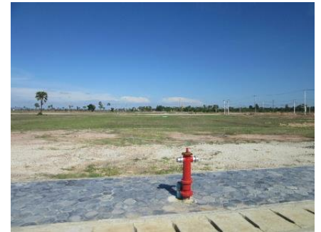
Water hydrant (Phnom Penh SEZ, Cambodia)
