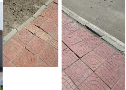
Sidewalk tiles are laid without firm foundation and already need repair
