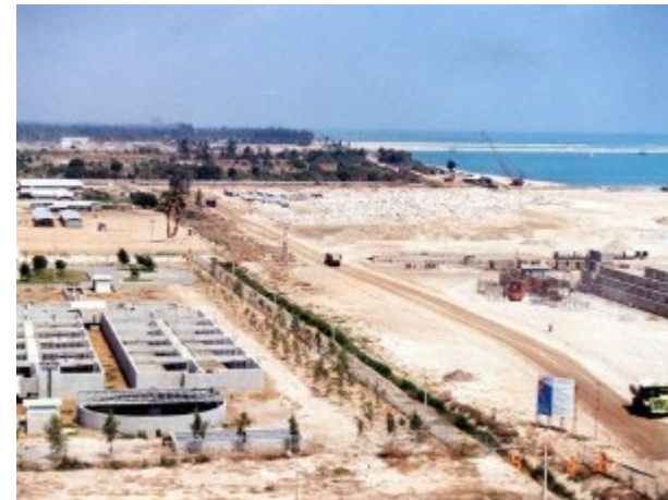
Construction site of Map Ta Phut Industrial Complex in early 1990s (Photo credit: JICA)
